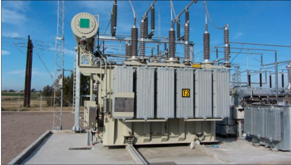
Figure 2. Picture of a conventional and typical 130/20 kV 40 MVA power transformer unit. A 63 MVA unit is physically slightly larger. [Ulf Lager E.ON Elnät Sverige AB]
