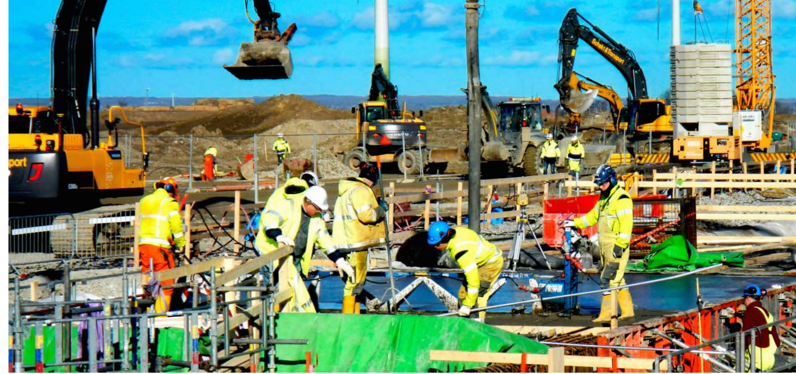
Construction workers casting a section of the Accelerator tunnel concrete vault. (Photo: ESS)
