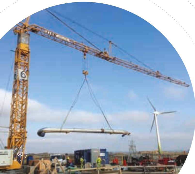
First installation: the Accelerator's cryogenic venting pipe
